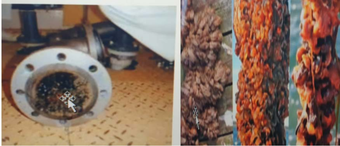
Fig. 9 Mucilage effects on the vessels engine cooler system filters.
